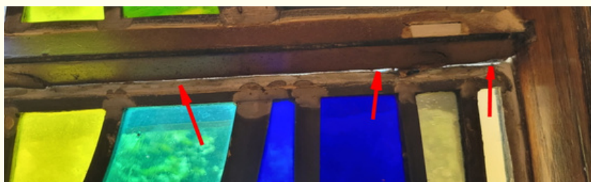
Central "Christ" window showing gaps due to lower glass panel sinking into the sill below.
