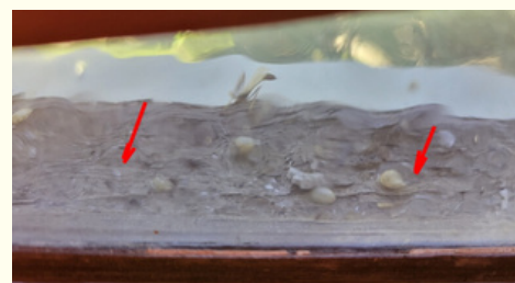
Looking through the glass of central "Christ" window - woodwork in need of repair & replacement.
